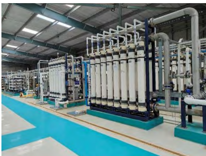
Ultra-pure water generation plant at Unit II
