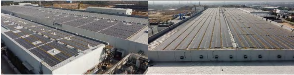
6.61 MW solar rooftop plant
